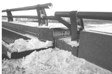
Paseo Bridge after dropping 9 inches
