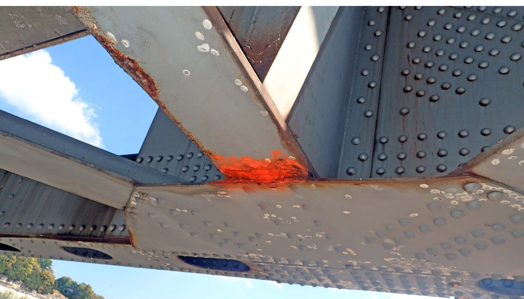
L0962 I-70 Cooper Floorbeam L16'L16' East End Bottom Flange Heavy Section Loss 10-2-17
