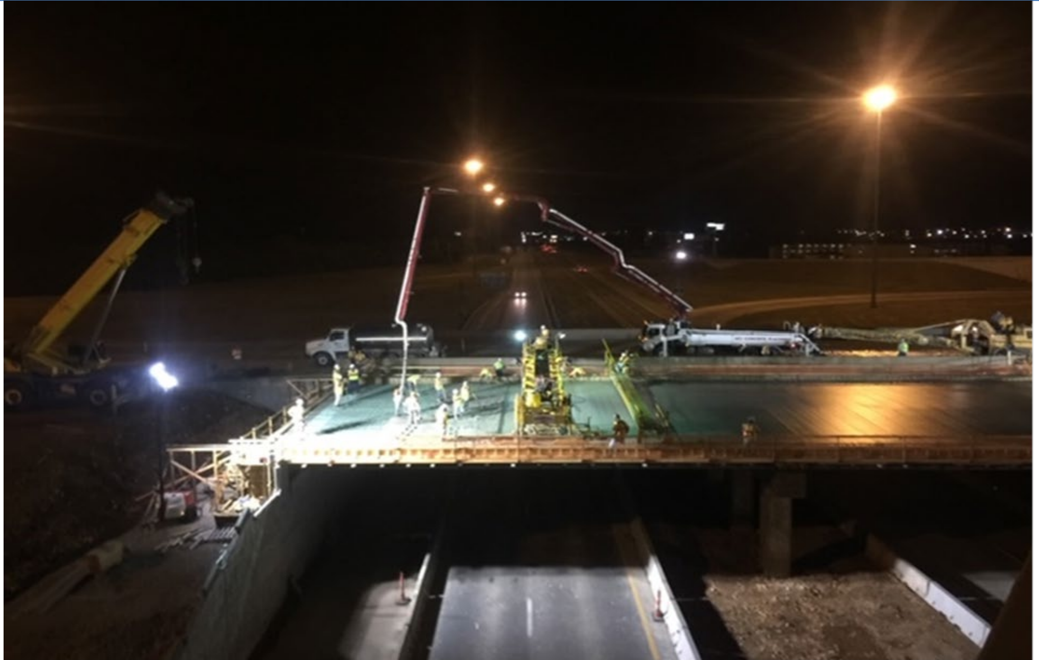
Crews reconstructing a bridge over I-44. Crews work at night to reduce impact to I-44 traffic. MoDOT is investing over $81 million to replace or rehabilitate over 50 rural bridges directly impacting I-44 in Southwest Missouri.
