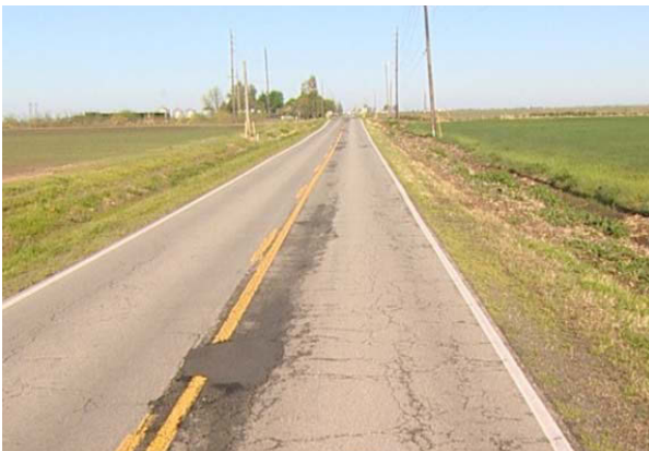
Before (Poor Condition Route)
