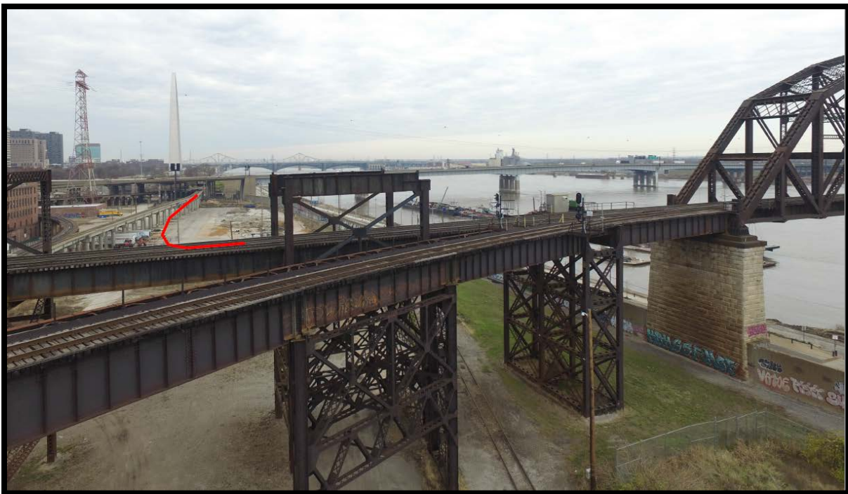
Figure 11 -- Not Feasible to Connect to North-South Route due to Highway Clearances, Grade, and Curvature
